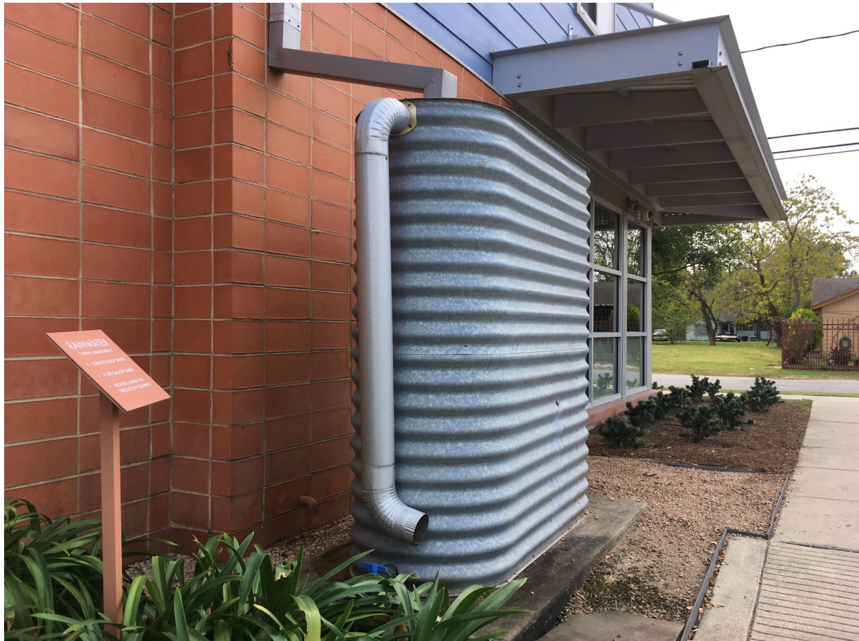
Rain cistern, New Hope Sakowitz Residence, Houston
